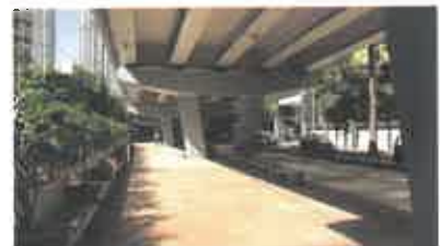
↖ ↑ ↗ The designed space under the flyover is a wide open place with an assembly of benches, planters, and safety buffers
